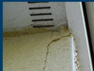
No mesh applied at return to reveal
