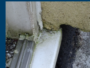
No return bead to cill - worn away as a consequence
