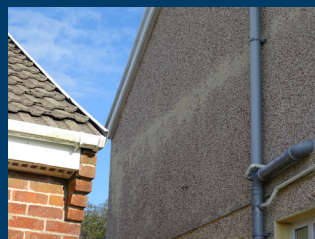
Application of dash finish poorly applied
