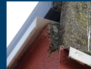
Terrible detailing exposing the system to the elements
