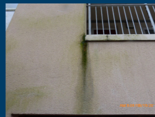
Beads not extended far enough across opening
