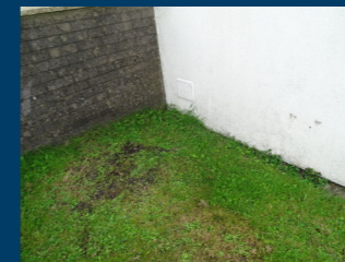
Poor design i.e. not left enough room at base for maintenance and grass cutting - could be hit with a mower
