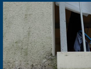
Copings not extended across opening
